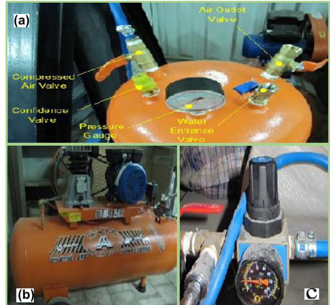
Pressure vessel a) Cylindrical tank a) installed equipment
